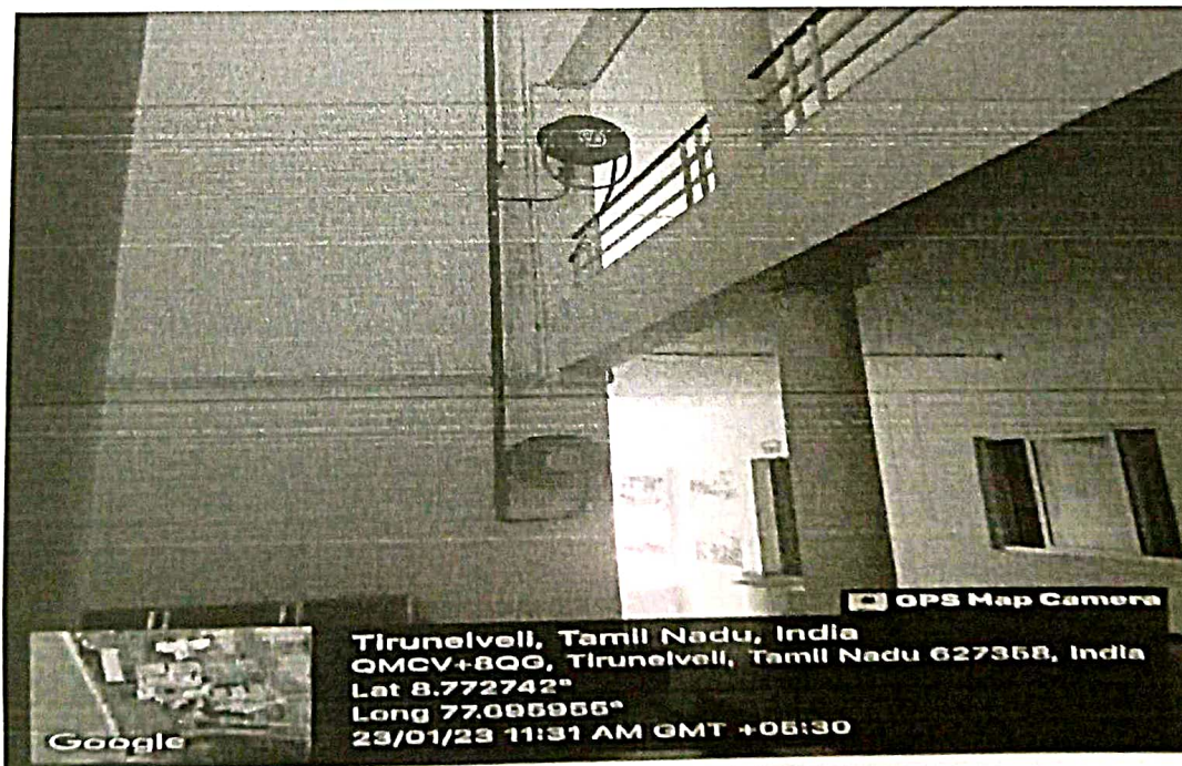
7.1.2 (a) 3. Fire Safety Pipeline
