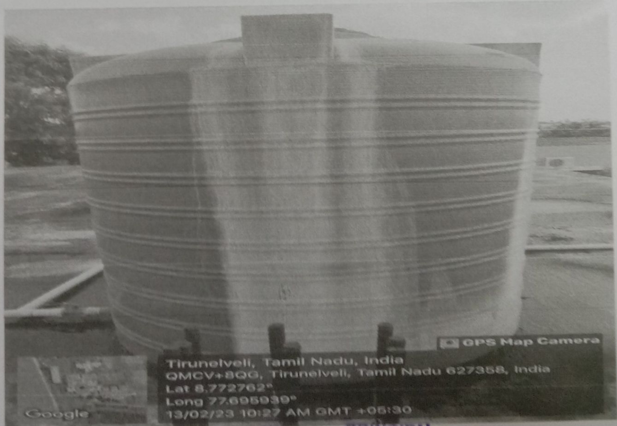
Figure 4: Water tank in OSE Block
